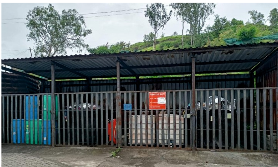
Photo: Hazardous Waste Storage
